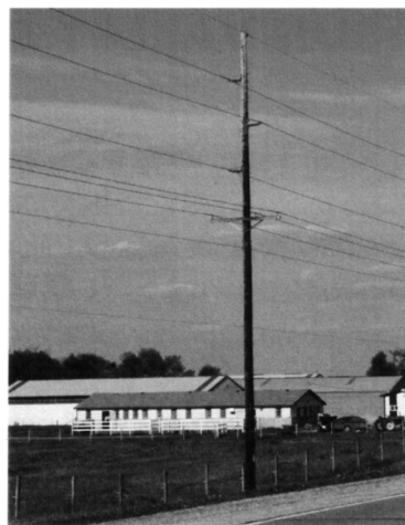
A slightly taller pole is used when electric distribution lines share the same structure as a 69-kV line.
